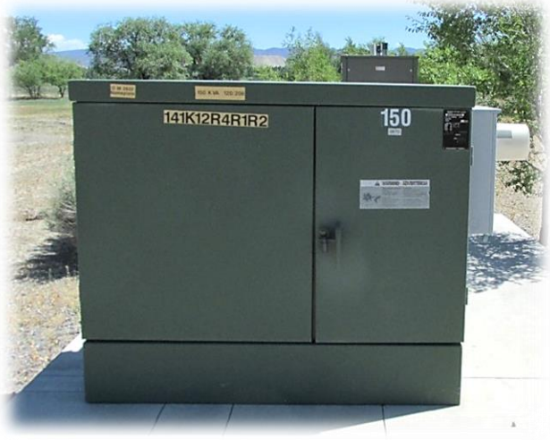
150 KVA 3-Phase transformer
