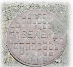
8" sewer main & tap installed. Sewer line inside the development is owned by the developer
