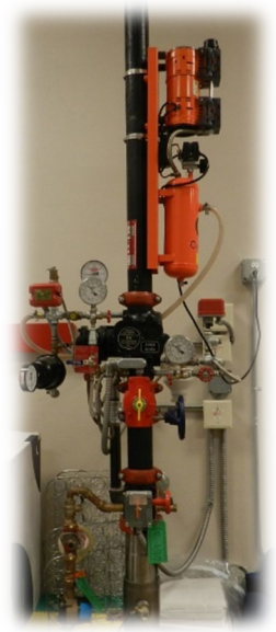
Fire suppression system
