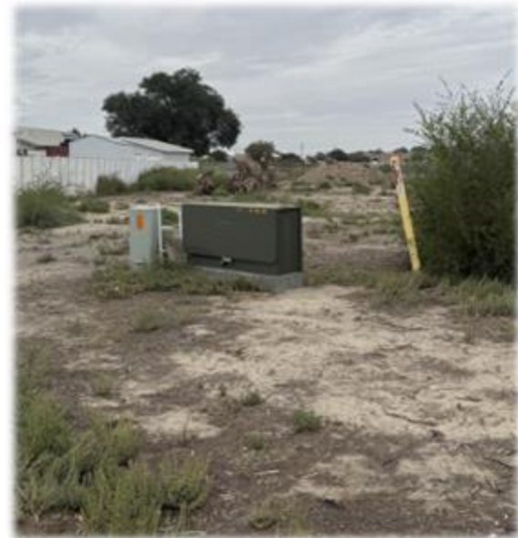
Power transform is the adjacent lot but can be accessed thru utility easement
