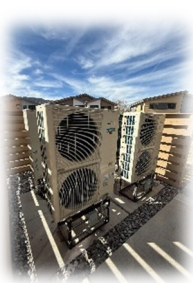
Each unit has their own HVAC
