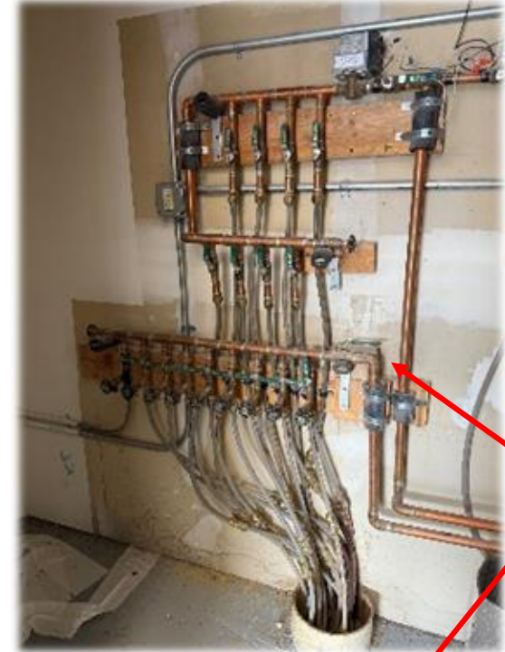
In Floor Heat System for Units A, B, C & D are in a closet on the back wall of Unit C
