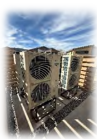
Each unit has their own HVAC
