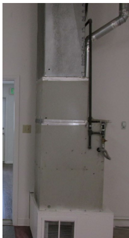
Forced Air Conditioning and Heat
