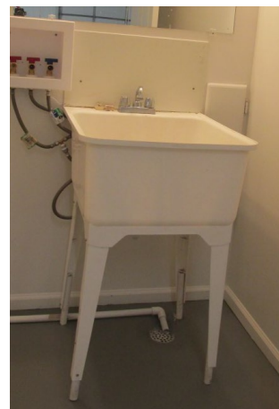
Utility Sink in Bathroom
