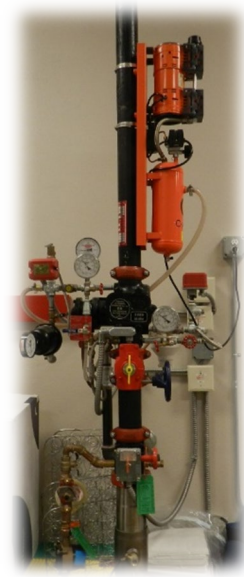
Fire suppression system
