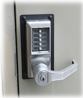
Keypad on front door, Unit 103
